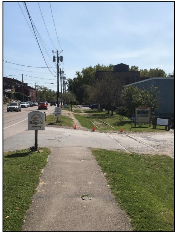
Photo 6-4: Existing Sidewalk Discontinuities
