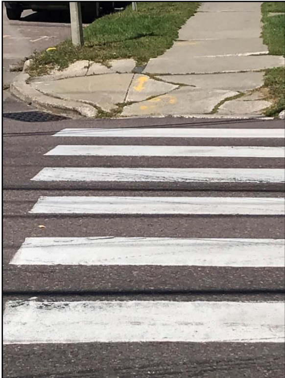
Photo 6-2: Numerous deficient sidewalk access ramps
