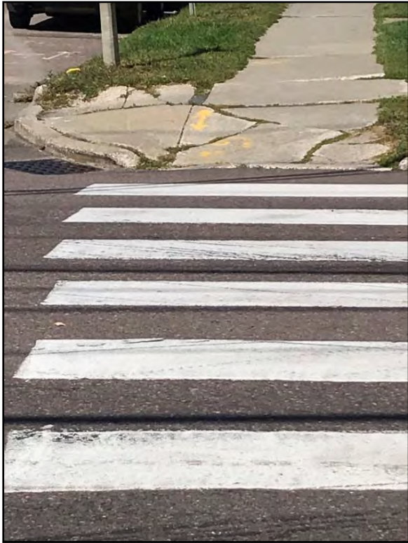
Photo 6-2: Numerous deficient sidewalk access ramps
